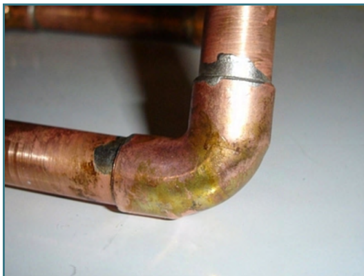
Copper pipes joined by lead solder.
