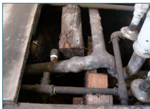
Example of lead pipes in a plumbing system.
