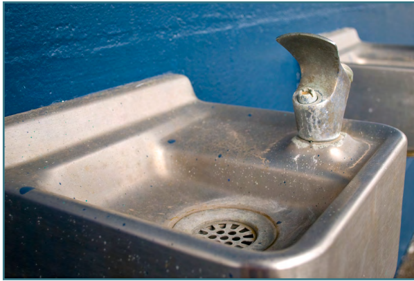
Lime build-up on mouthpiece and protective guard of drinking fountain.
